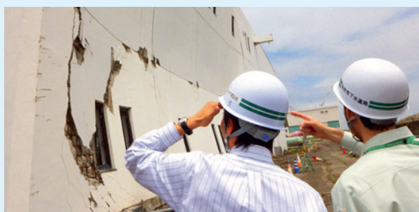
Wastewater treatment plant damaged by the 2011 tsunami.
